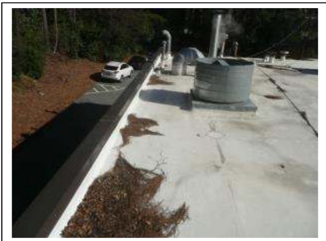
Debris on the roof- mostly pine straw
